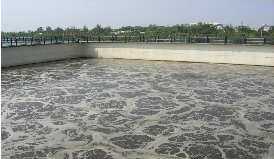
Picture: Showing Activate Sludge Process (Diffuse Aeration)
